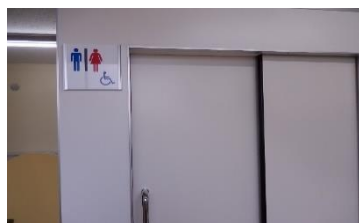
Handicap accessible multipurpose bathroom
